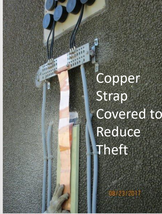
External Ground Bar Bonded
